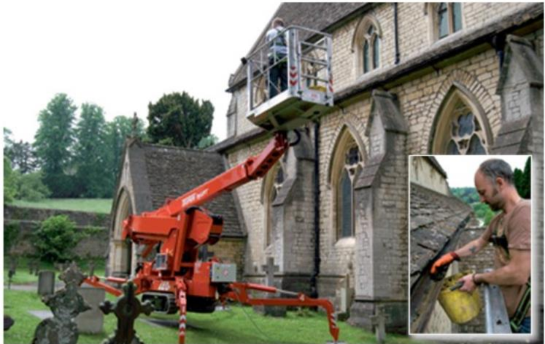
Rob Forrester of Forrester Access clears the gutters at Priory Church of the Annunciation, Inchbrook, Stroud for GutterClear, Maintain our Heritage's scheme in Gloucestershire (Photos: Jonathan Taylor)
